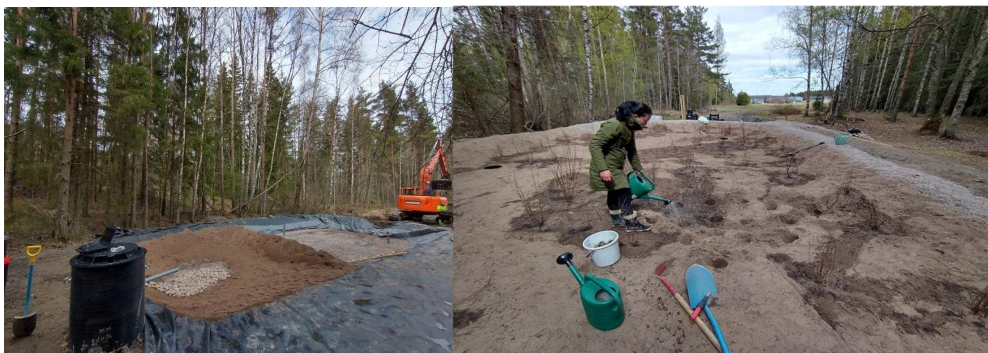
Installation of the filter medium (left) and watering of newly planted vegetation at the Lieto pilot (right).
