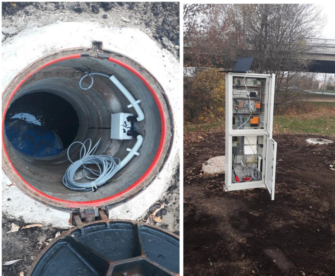
Inside of the treatment solution with sensors, switchboard and controller
