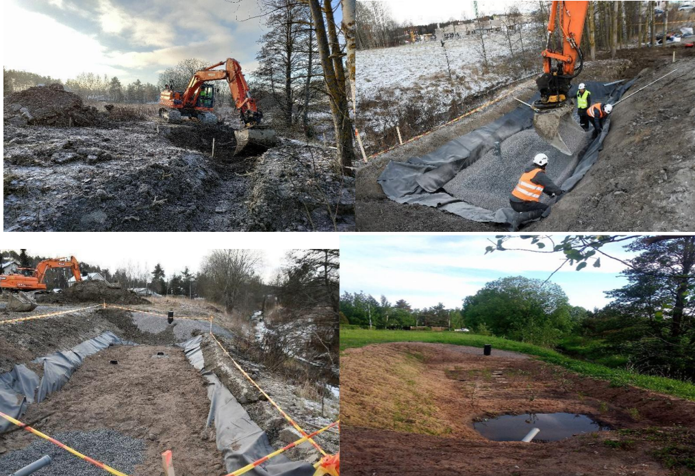
Construction of the Turku pilot site in December 2021 (top) and the ready bioretention basin in May 2022 (bottom right).
